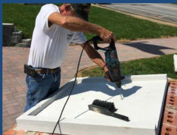
Document Tray Being Placed and Secured DOCUMENT TRAY BEING PLACED ON TOP OF FOUNDATION SUPER-STRUCTURE
