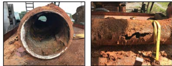
Failed Ductile Iron Pipe – 9 years old.
