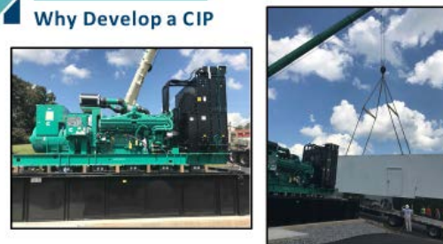
Water Treatment Plant – Backup Generator
