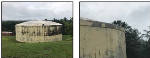
Water Treatment Plant – Finished Water Clearwell
